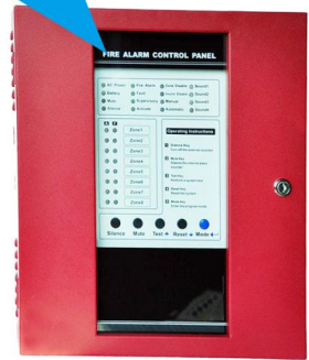
Fire alarm system
