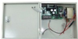
Access control power supply EA-39
