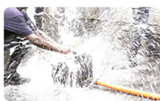
Water pipe cracking leaks
